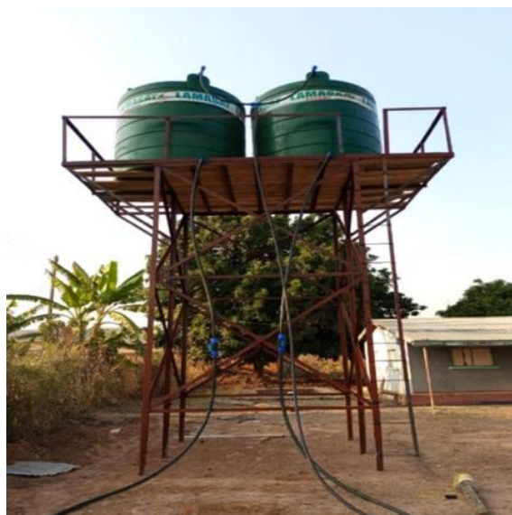
Water tanks connected to irrigation pipes.
